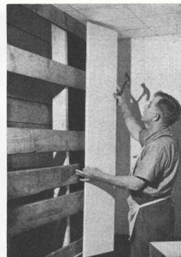
Walls. Insulation board planks, 12 inches wide, were nailed to furring at edge. Next board conceals nails
